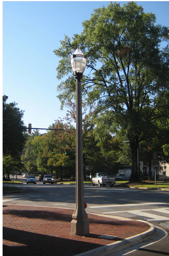
ACORN LIGHTING FIXTURE
