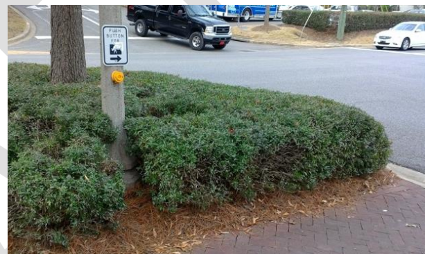
FIGURE 10: NON-COMPLIANT PEDESTRIAN SIGNAL (DUE TO EXCESSIVE HORIZONTAL REACH AND NON-COMPLIANT DISTANCE FROM CURB/PAVEMENT)
