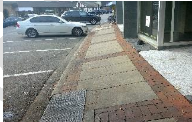
FIGURE 2: NON-COMPLIANT SIDEWALK (DUE TO CROSS SLOPES EXCEEDING 2%)
