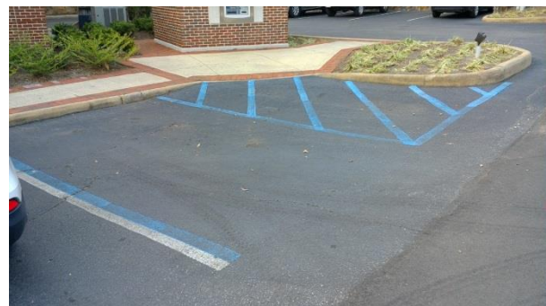
FIGURE 8: NON-COMPLIANT ON-STREET PARKING AREA (DUE TO SLOPES IN EXCESS OF 2% AND LACK OF SIGNAGE)
