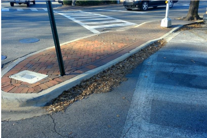
FIGURE 11, TO LEFT: NON-COMPLIANT REFUGE ISLAND (DUE TO NON-COMPLIANT NARROW WIDTH AND LACK OF DETECTABLE WARNING SURFACES)
