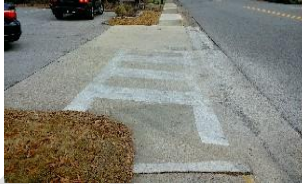
FIGURE 6: NON-COMPLIANT CROSS WALK (DUE TO EXCESSIVE CROSS SLOPE, NEEDS RE-STRIPING TO CONFORM TO CURRENT MUTCD STANDARDS)
