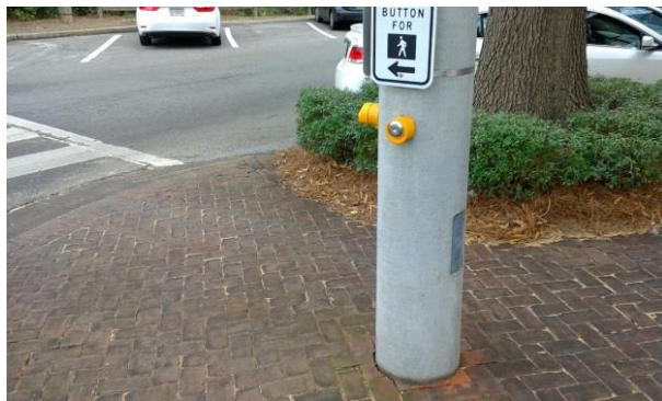
FIGURE 9: COMPLIANT PEDESTRIAN SIGNAL
