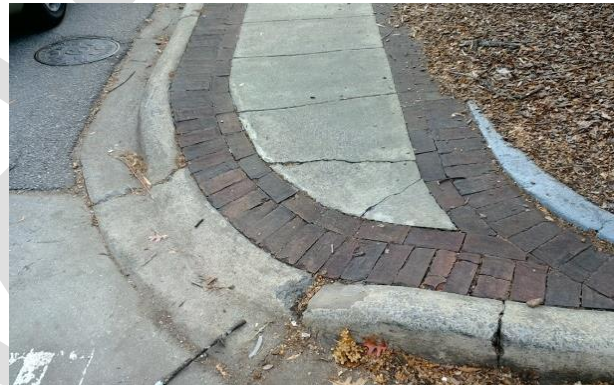
FIGURE 4: NON-COMPLIANT CURB RAMP (DUE TO EXCESSIVE SLOPES, A NON-COMPLIANT WIDTH, AND NO DETECTABLE WARNING SURFACES)
