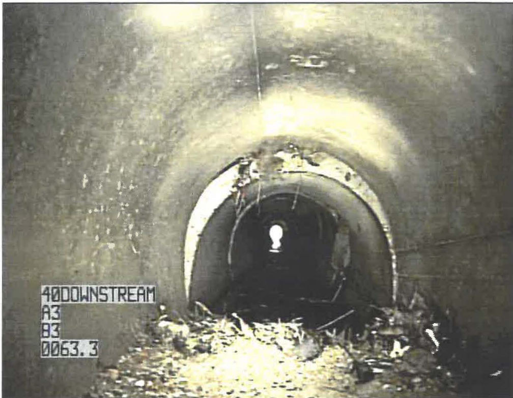
Top picture before partial cleaning looking upstream. Lower picture looking downstream after removal of the log.
