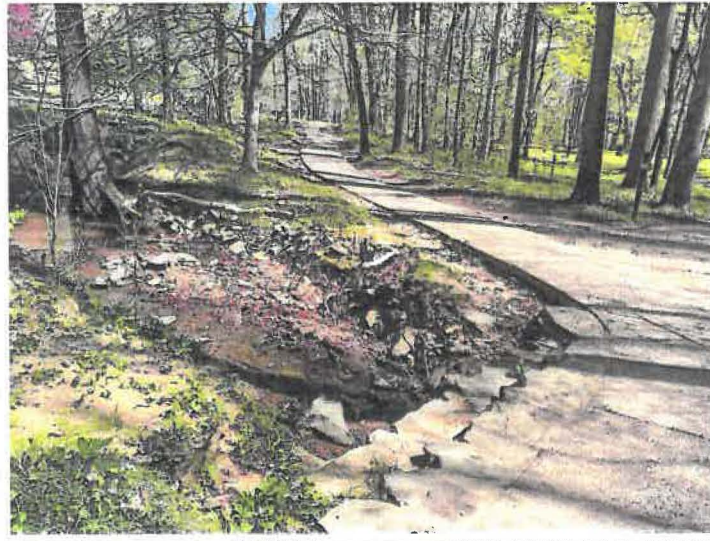
Stream Bank Erosion
