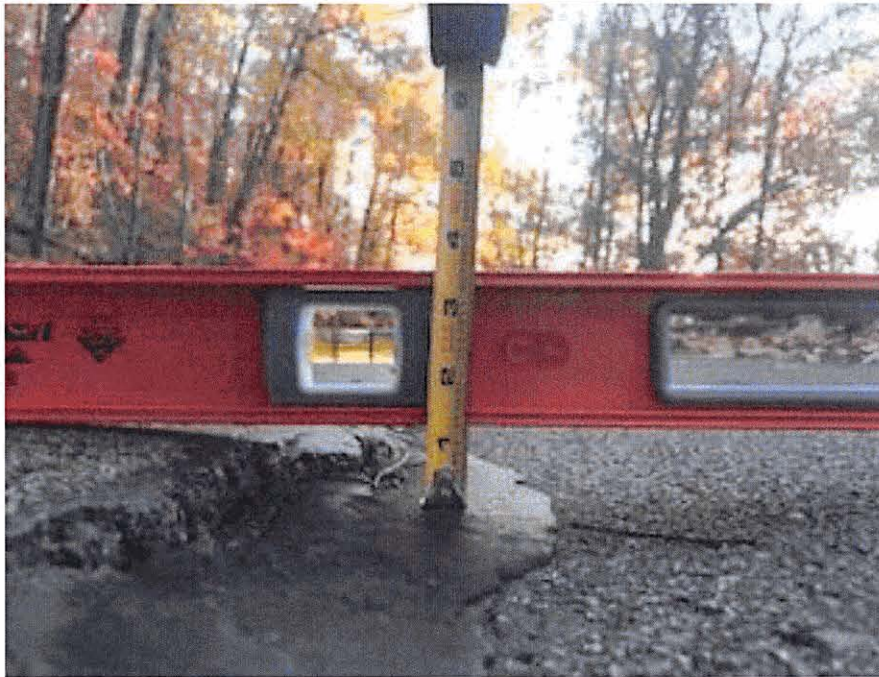
Photograph 3, Area 1: Rutting Depth of 1.5"
