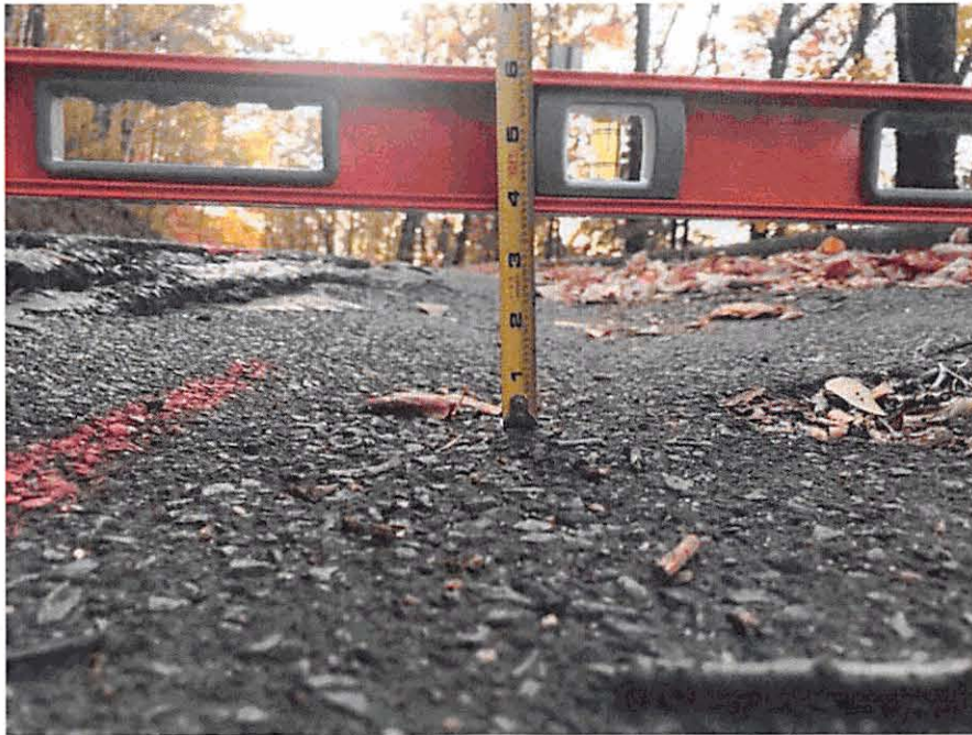
Photograph 9, Area 4: Rutting Depth of 3.75"
