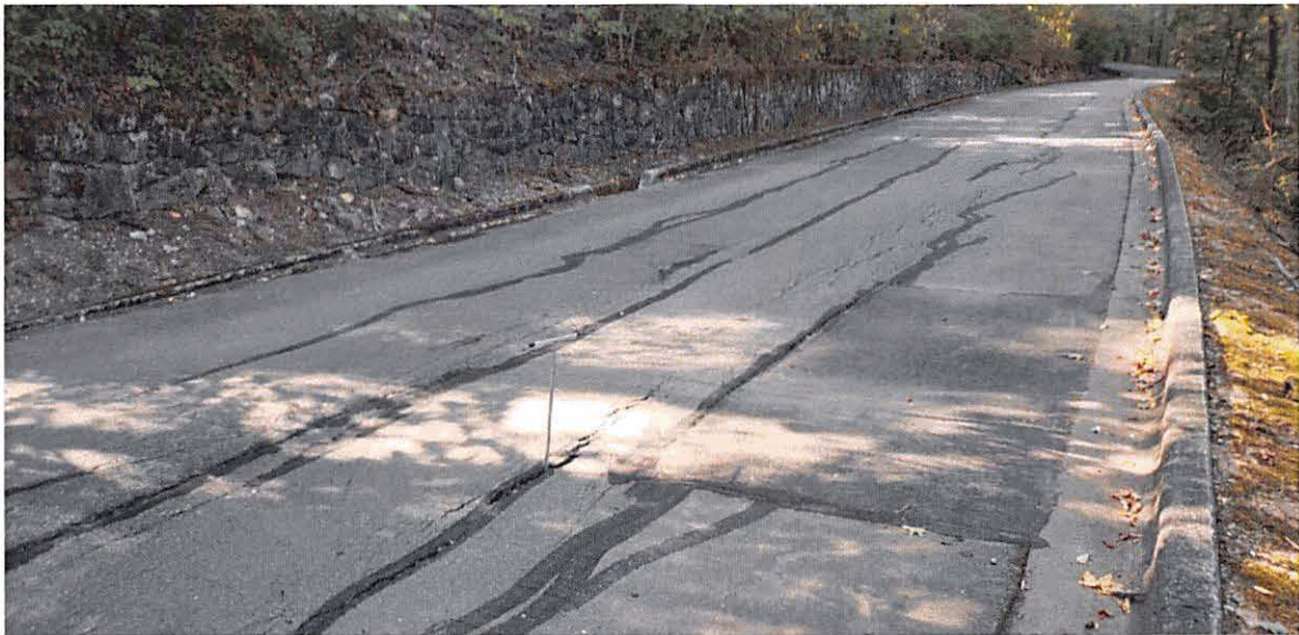
Figure 2.3.2 – Typical View of Pavement Rutting and Tearing, Area of Prior Crack Seal is Visible
