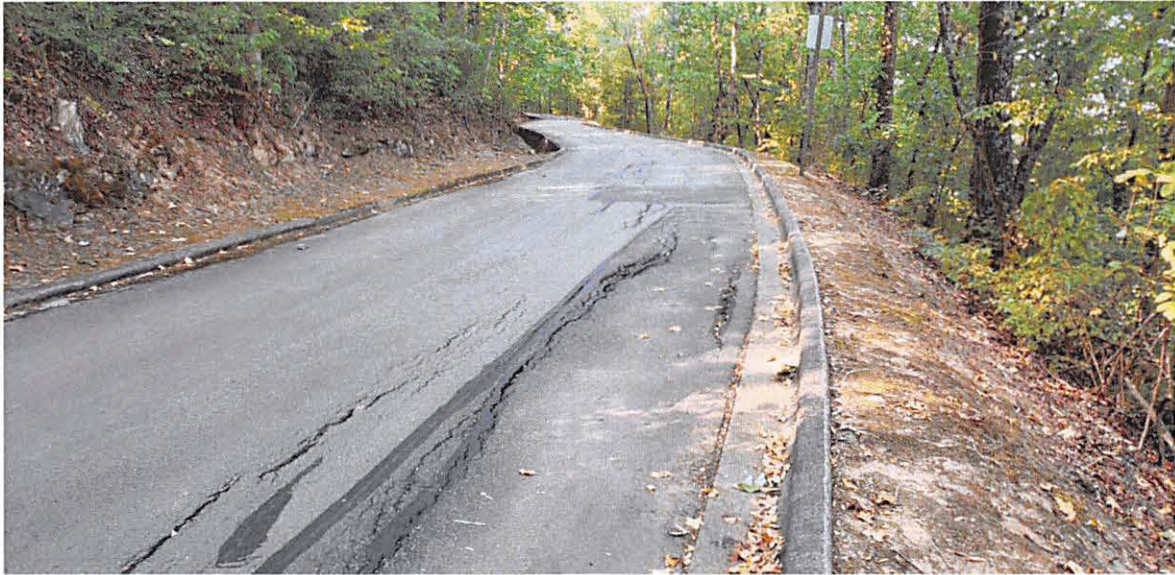
Figure 2.3.1 – Typical View of Pavement Rutting and Tearing
