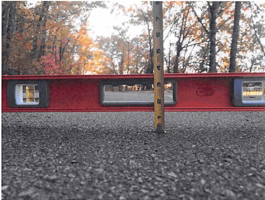
Photograph 5, Area 2: Rutting Depth of 1.5"
