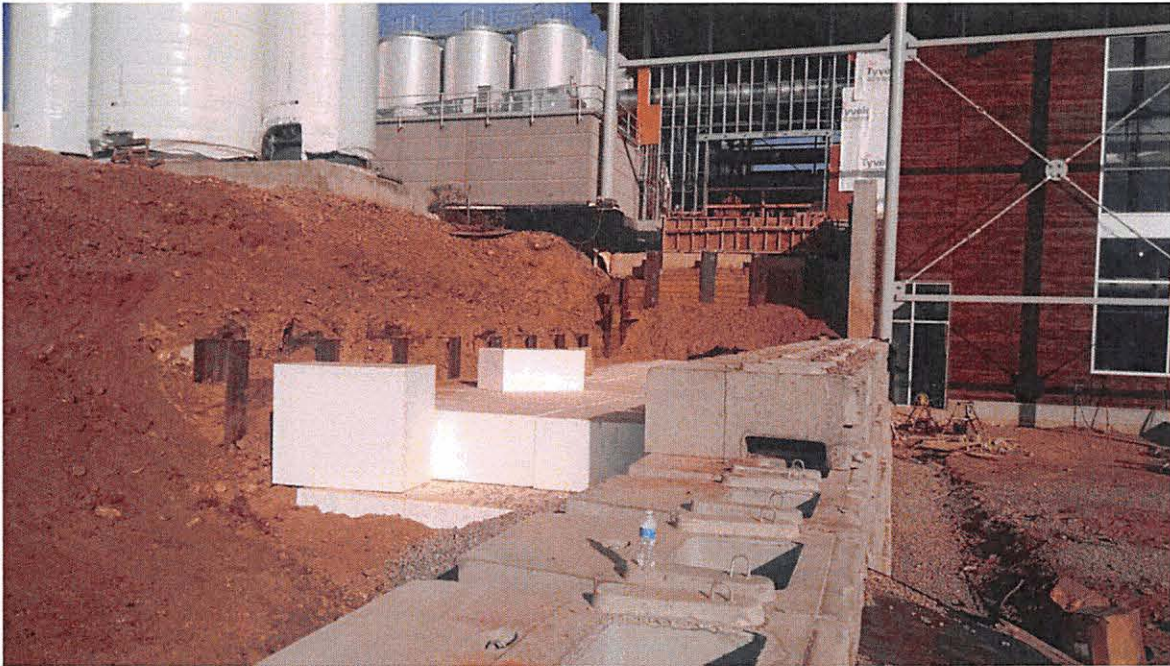
Figure 5.1.1 – Example View of EPS Backfill Behind Gravity Retaining Wall (from Author's Personal Photos)
