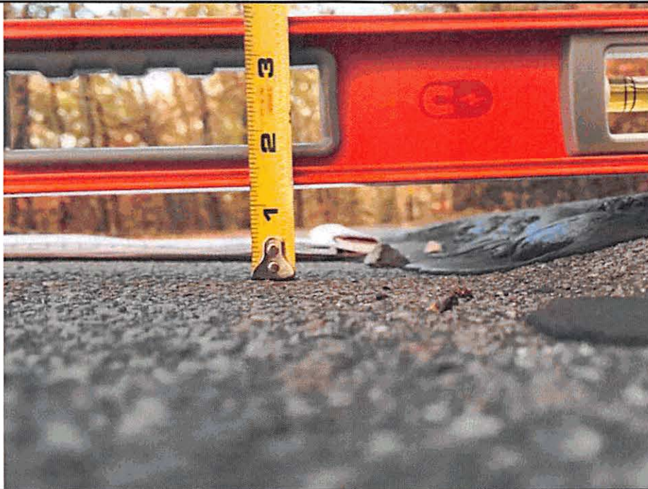
Photograph 7, Area 3: Rutting Depth of 1.5"
