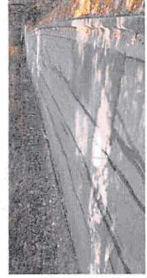
Figure 2.3.2 – Typical View of Pavement Rutting and Tearing, Area of Prior Crack Seal is Visible
