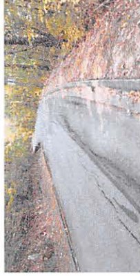
Figure 2.3.1 – Typical View of Pavement Rutting and Tearing
